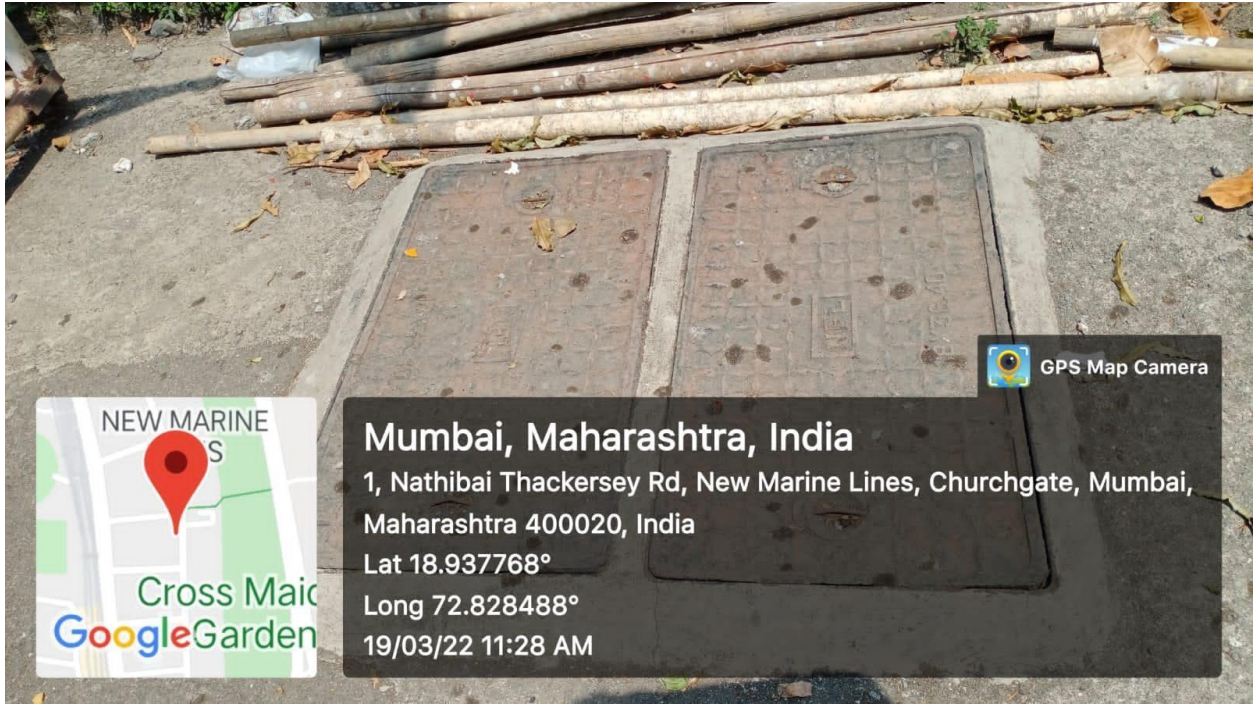
Rain water harvesting system at SNTWU, Churchgate Campus
